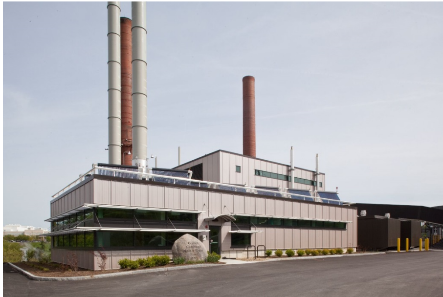
CHP plant at Cornell University
