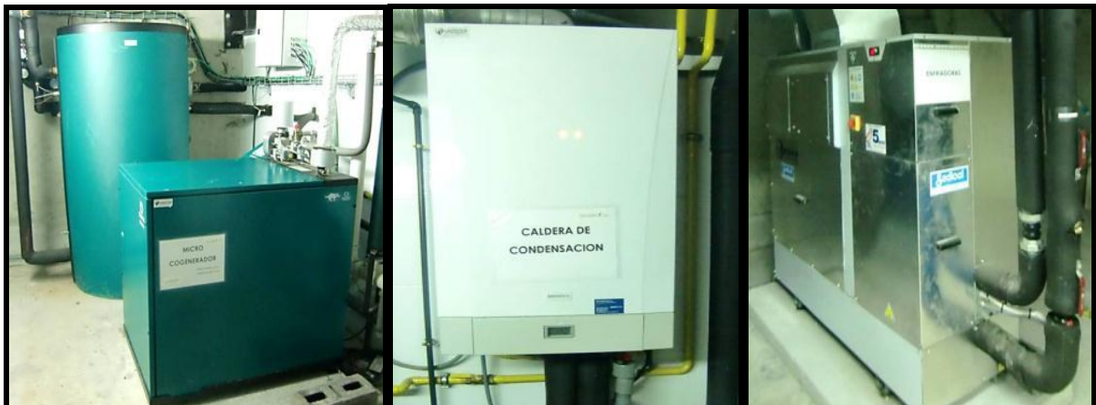
CHP+ Storage tank, Boiler and Chiller installed in KUBIK
