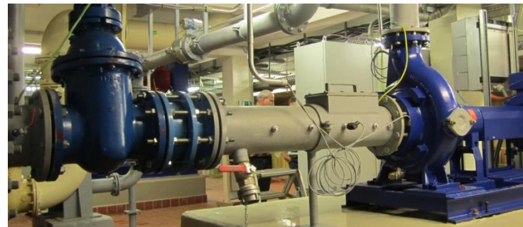
Teststands in laboratory and in wastewater pumping station Berlin-Lichtenberg
